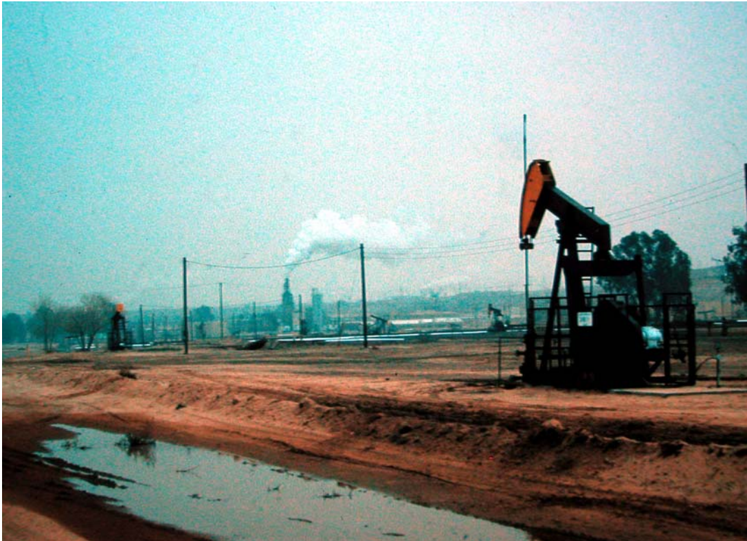
Figure 5. Secondary recovery is used in most oil fields to enhance production. Water is injected commonly and is used in Saudi Arabian fields, while steam shown here is used too. The steam plants, shown in the distance venting steam, pump steam into the oil-bearing strata and force the oil to other wells nearby where it is extracted. The technique works on heavy crude and fields that are somewhat depleted. See http://www.heavyoilinfo.com/thermal . J. H. Lipps image, 1960.
